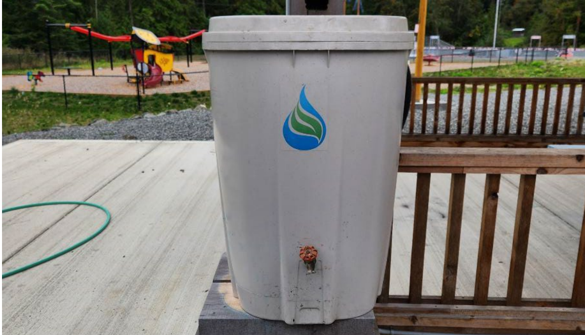
Image 7: Existing Rainwater Capture Tank by Talking Circle, Malahat Nation
